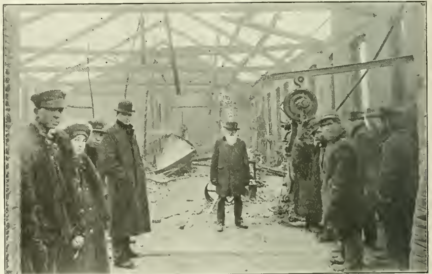
MACHINE SHOP AT ELKHART, IND., DESTROYED BY FIRE. L. S. & M. S.
